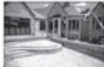
Construction continues in July on the largest pool project to date for Agile Aquatic of Cedar Rapids. The in-ground infinity pool also has a spa, a waterfall, a moat and an island barbecue. (Geoff Stellfox/The Gazette)
